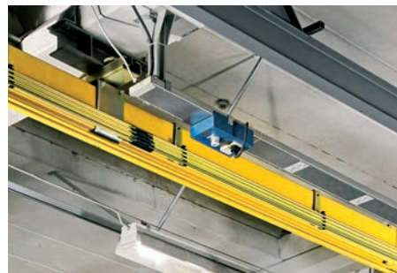
Enclosed Conductor Power System
